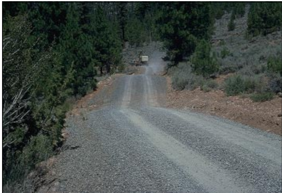
Photo 7.1 Design roads that move water rapidly off the surface of the road and minimize water concentration with the use of rolling grades and outsloped, insloped, or crowned roads.
